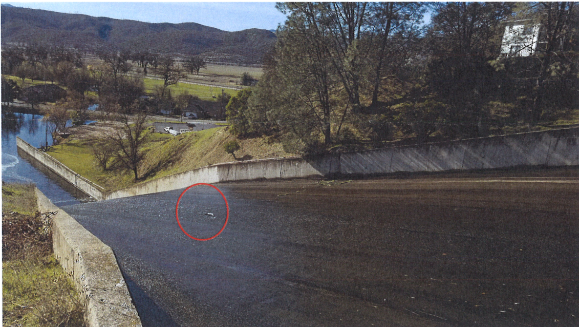
Photo 2: View of spillway chute. Small voids were observed, one is circled.
