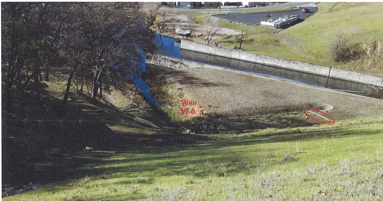
Photo 4: Collector ditch for outfall drain weirs, designated W1 through W5, located at toe. The CMP drainage pipe for the seepage band is circled. Approximate location of W6 is noted.
