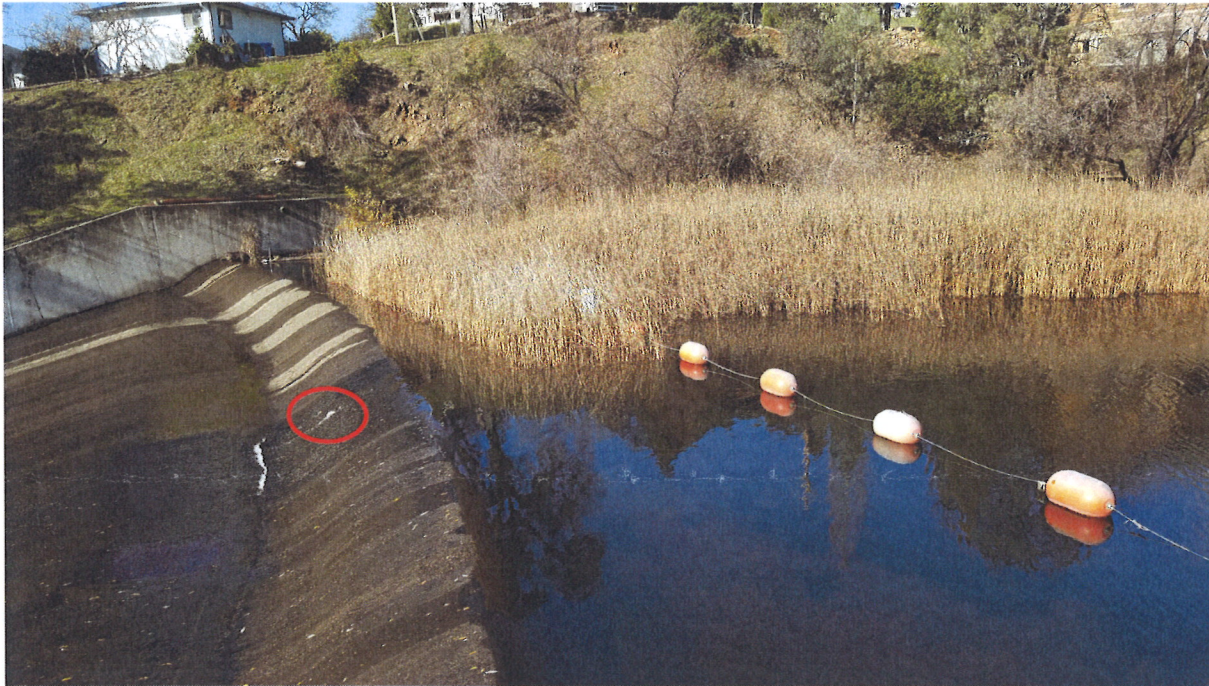
Photo 3: Another small void in the spillway weir (circled). Note the dense Tule growth which needs to be removed.
