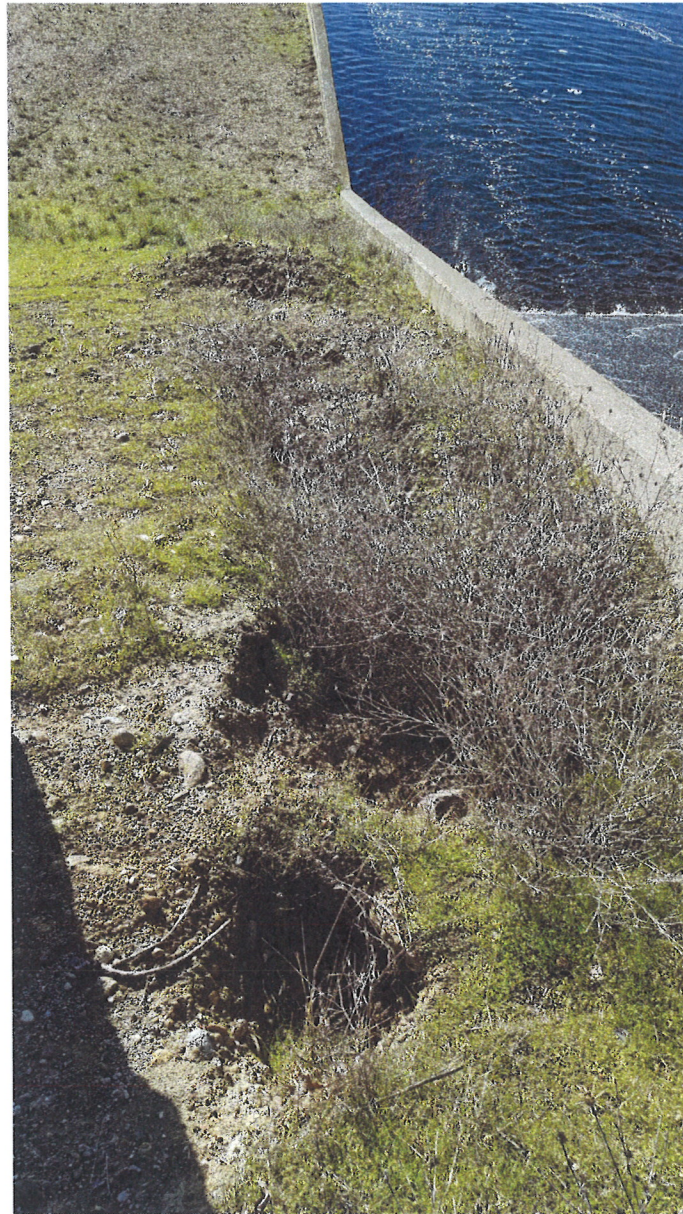
Photo 5: Large voids observed behind the left spillway wall. Other smaller voids were observed, but not photographed. All locations along the left wall were identified and discussed with the owner's representatives on site.
