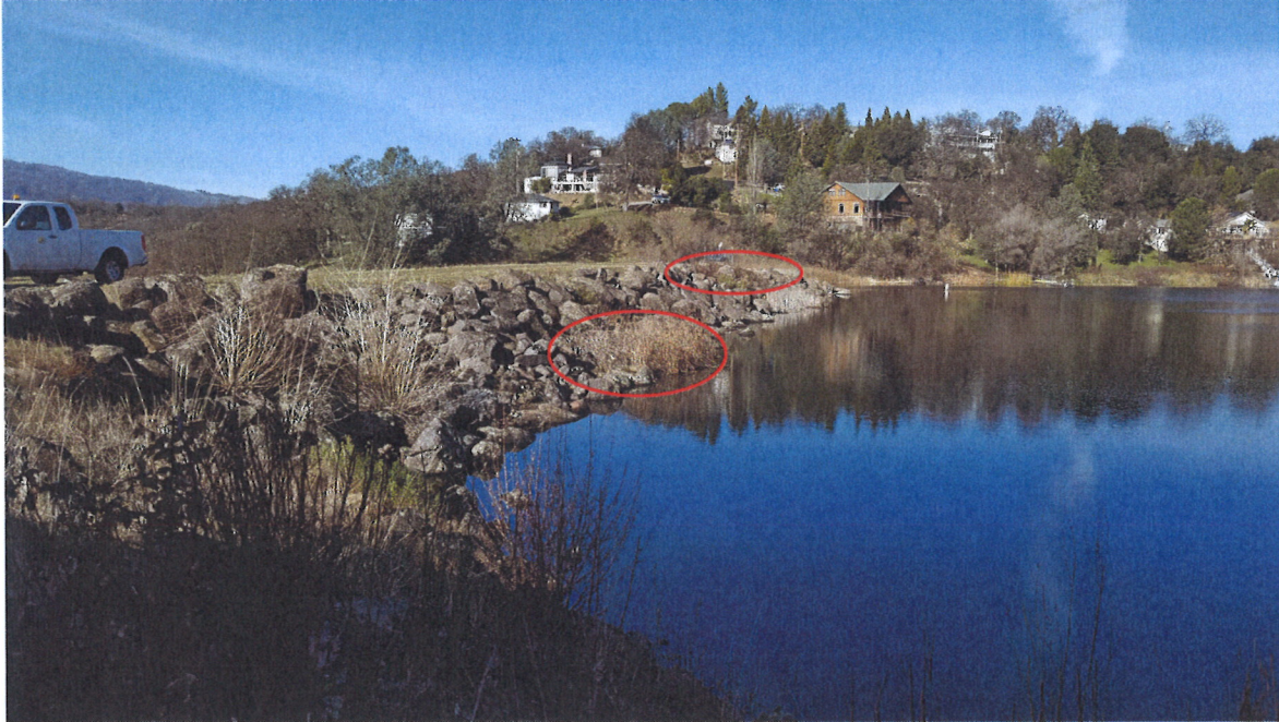
Photo 1: Upstream face of dam viewed toward the right abutment. Vegetation and berry vines are circled.
