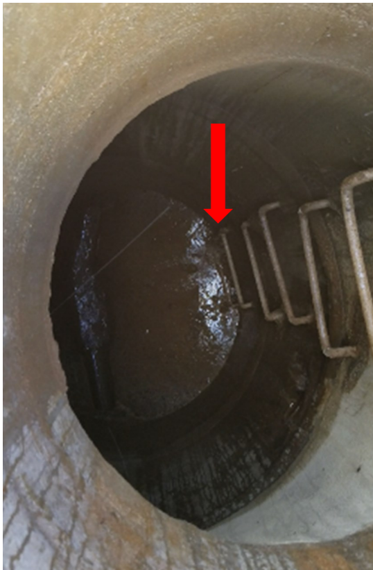
Manhole Inspections: Infiltration at the ladder
