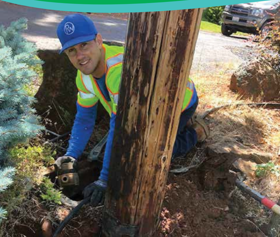
Water Treatment Operator 1 Blake Graham with Rancho California Water District works on a Paradise Irrigation District meter. Graham was among two crews recently sent by his Temecula-based district to assist PID in its recovery from last year's Camp Fire. At least a dozen ACWA member agencies have extended assistance to ACWA member PID since the fire.
