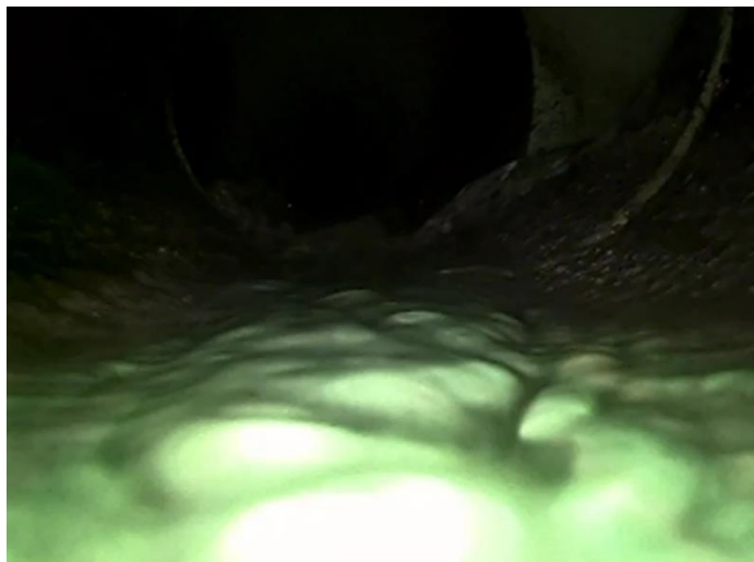
Cleanout intrusion from the main.
