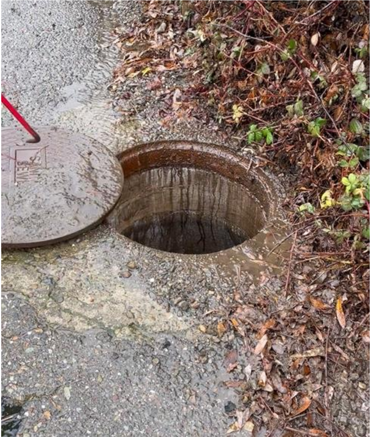
Figure 4: Manhole 9.0-3 with direct inflow stream flowing from uphill.
